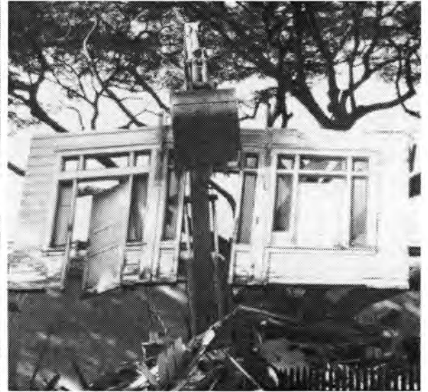
The last visible wall is picked up by the claw and about to be trashed to pieces.
