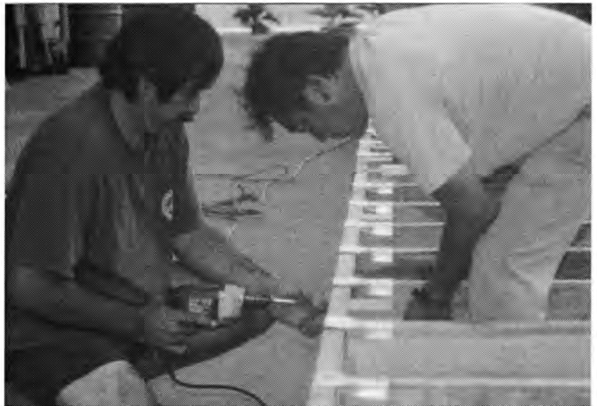
“Joe” Pacquing and Dennis Shiraishi assembling stage. The materials were donated by MIDPAC Lumber Company.
